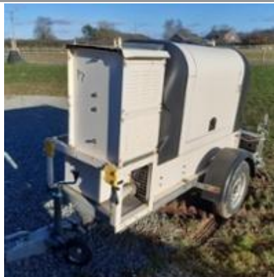
2005 14 KVA Diesel Generator
